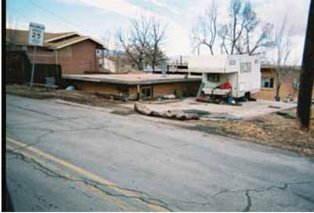
Lack of Property Maintenance
